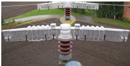
BCIC-1217-TR: Post Insulator application
