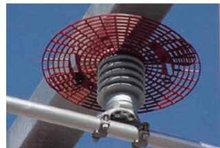
BISG-60/115-02 installed on bus support insulator
