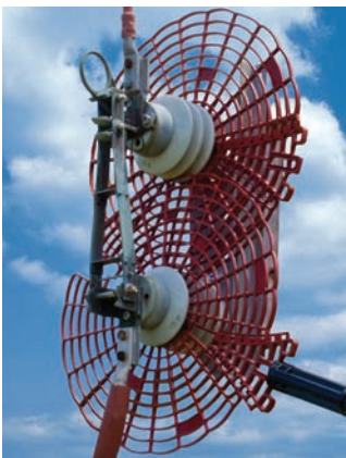
BISG-24 energized install
