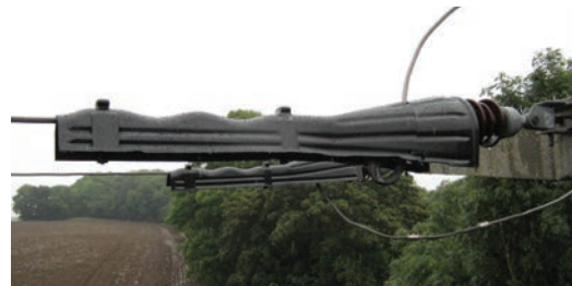
BCIC-TEN-01: Tension Insulator application
