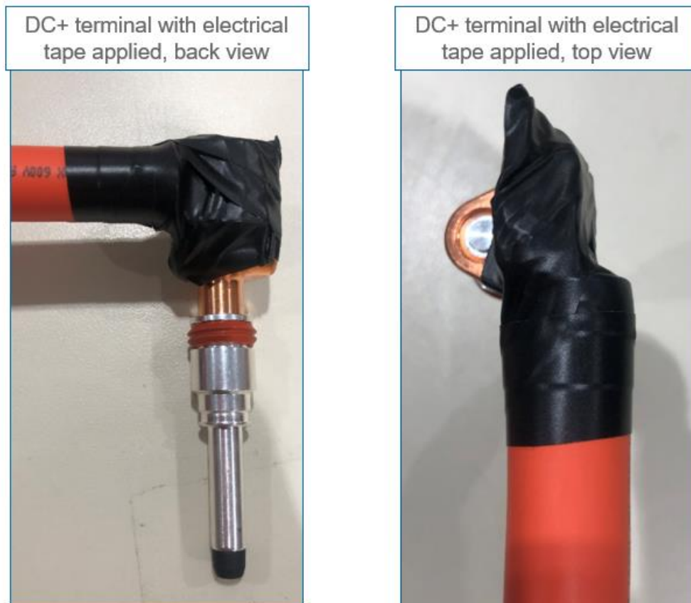
Figure 30: DC+ terminal with electrical tape applied
