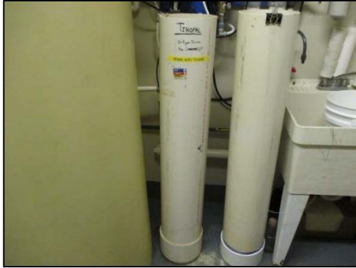
Figure 24 – 1m Test Vessel
