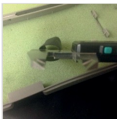
INCORRECT ID TUBING IS STRETCHED
