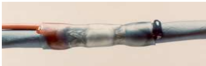
Unacceptable: Insufficient heat. Contour of solder perform is visible.
